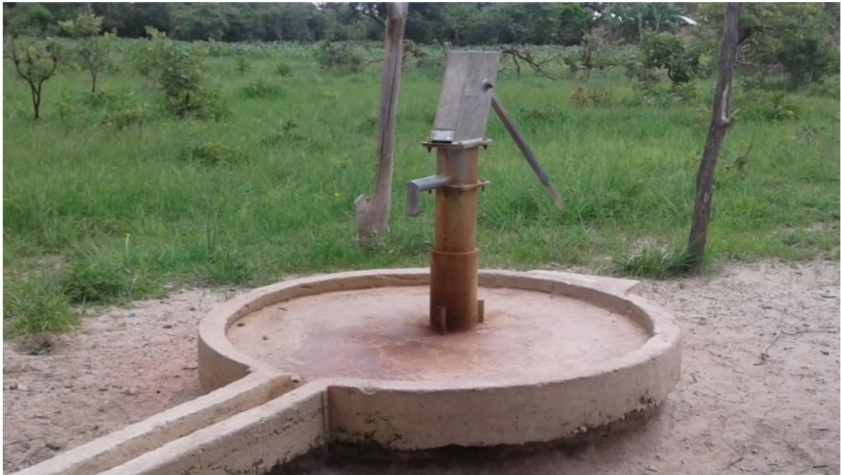
Picture 4: Rust stained pedestal and concrete apron at Shanyanga Village, Chongwe
