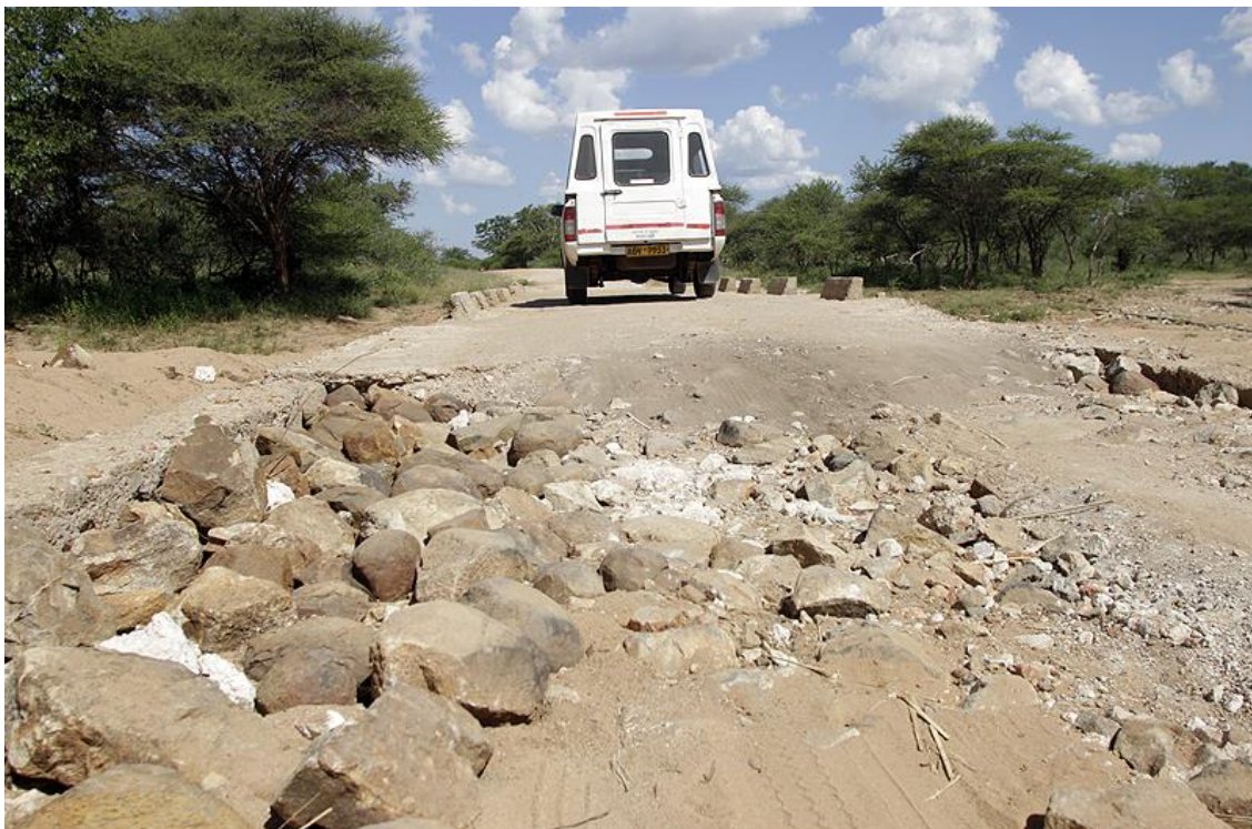
Figure 17: State of road in Mapisa, Matebeleland South
