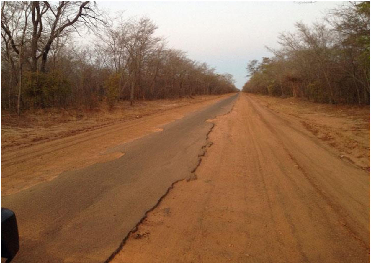
Figure 16: State of Bulawayo-Nkayi road
