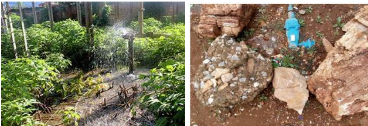
Figure 4.2: leakages and old pipes. Source: field survey, (2025)
