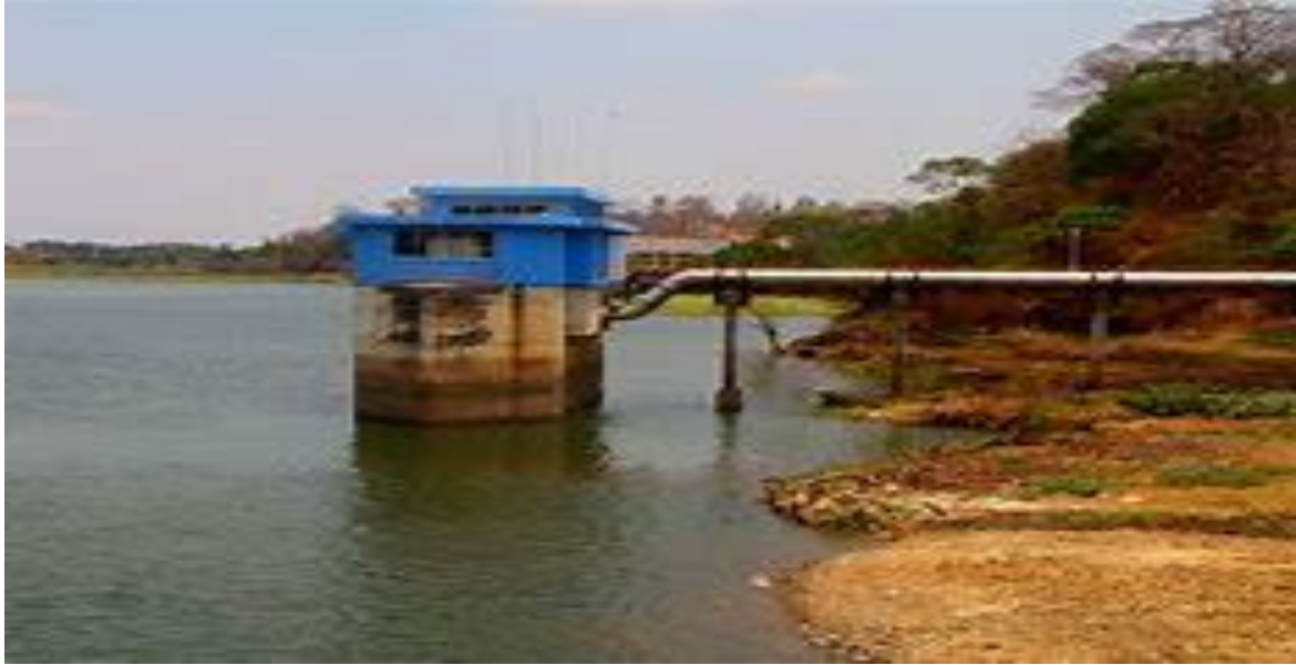
Figure 2.1: maintained water generating plant. Source: (LWSSC2025)
