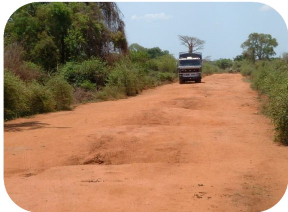
Figure 52: A road in Katete before OPRC (Source: Adapted from RDA, Report, 2009)
