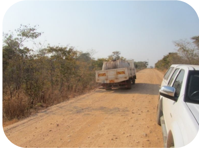
Figure 66: Large stones exposed on Ruyala road in Zimba
