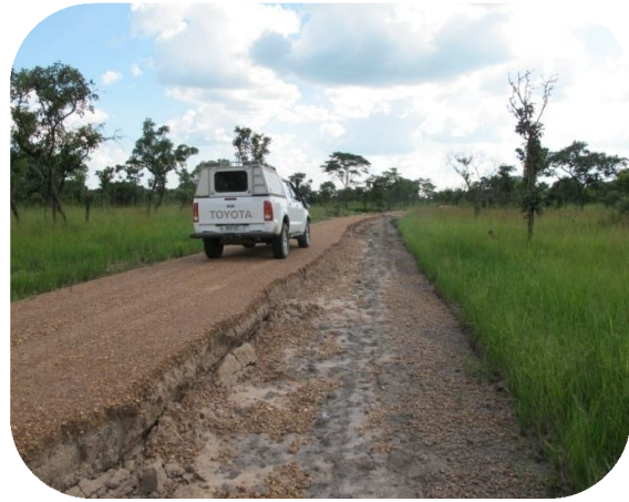
Figure 60: Washed out Spinal Road during 2012-2013 Rainy Season
