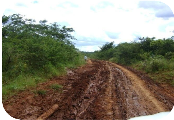
Figure 50: Chongwe to Chalimbana road before OPRC, 2009 (Adapted from RDA, Report, 2010)
