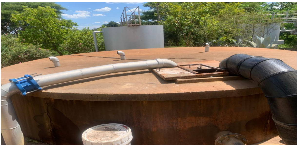
Figure 8: Showing the Chlorination Tank at NWWSSCL Water Treatment Plant
