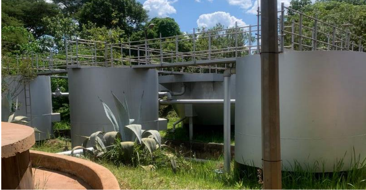
Figure 7: Showing filtration Chambers at NWWSSCL Water Treatment Plant
