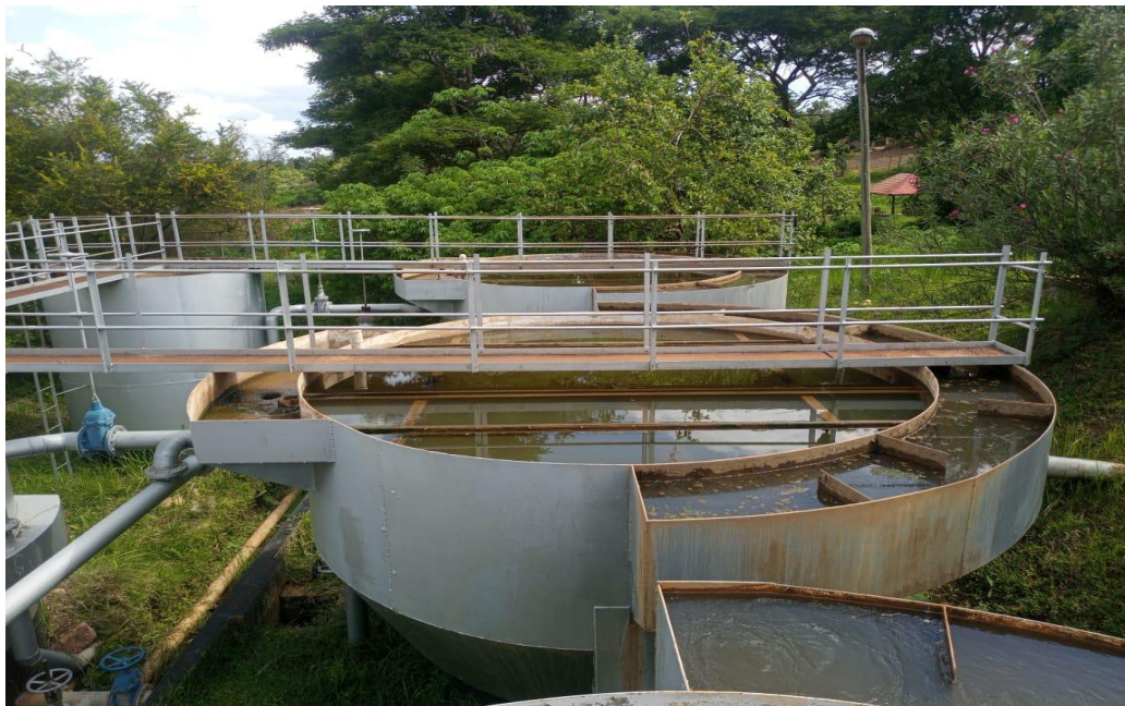
Figure 6: Showing the Sedimentation thickeners at NWWSSCL Water Treatment Plant
