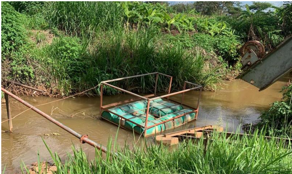
Figure 15: Raw water abstraction stage at the Water Processing Plant
