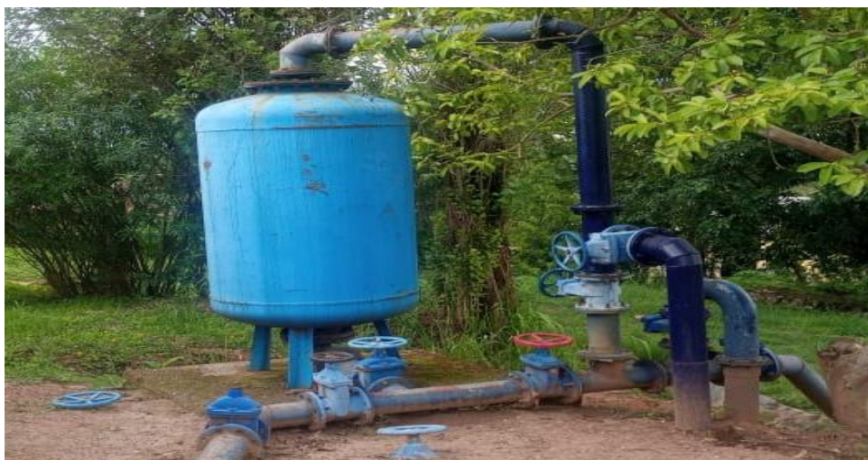
Figure 10: Showing the Pressure filter water treatment process at NWWSSCL Water Treatment Plant.
