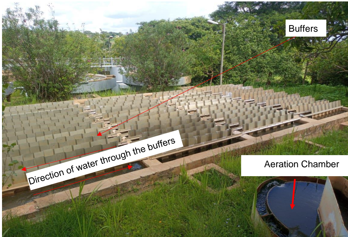
Figure 5: Showing the Flocculation chambers of NWWSSCL water treatment Plant
